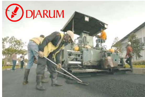
Application of 39,000 m 2 of plastic asphalt in Kudus, Central Java, with PT Djarum
